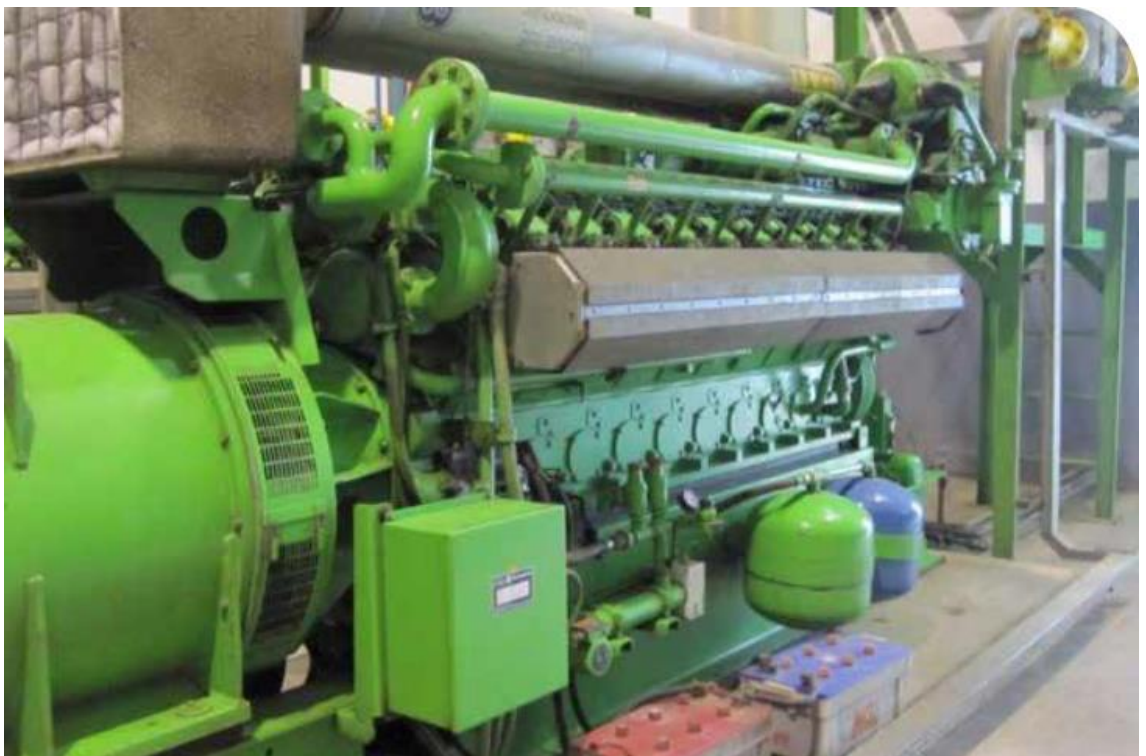
Figure 34. Example a Jenbacher 1 MW gas engine at Bantergebang (ref 2).
